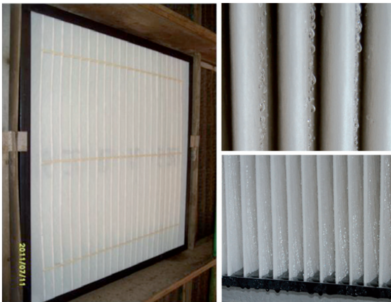
Fig. 5 - Water first coalesces then drains away from the downstream air flow
